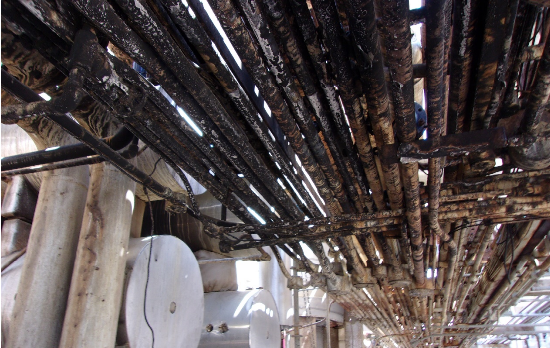
Figure 2. Damage to Overhead Piperack
