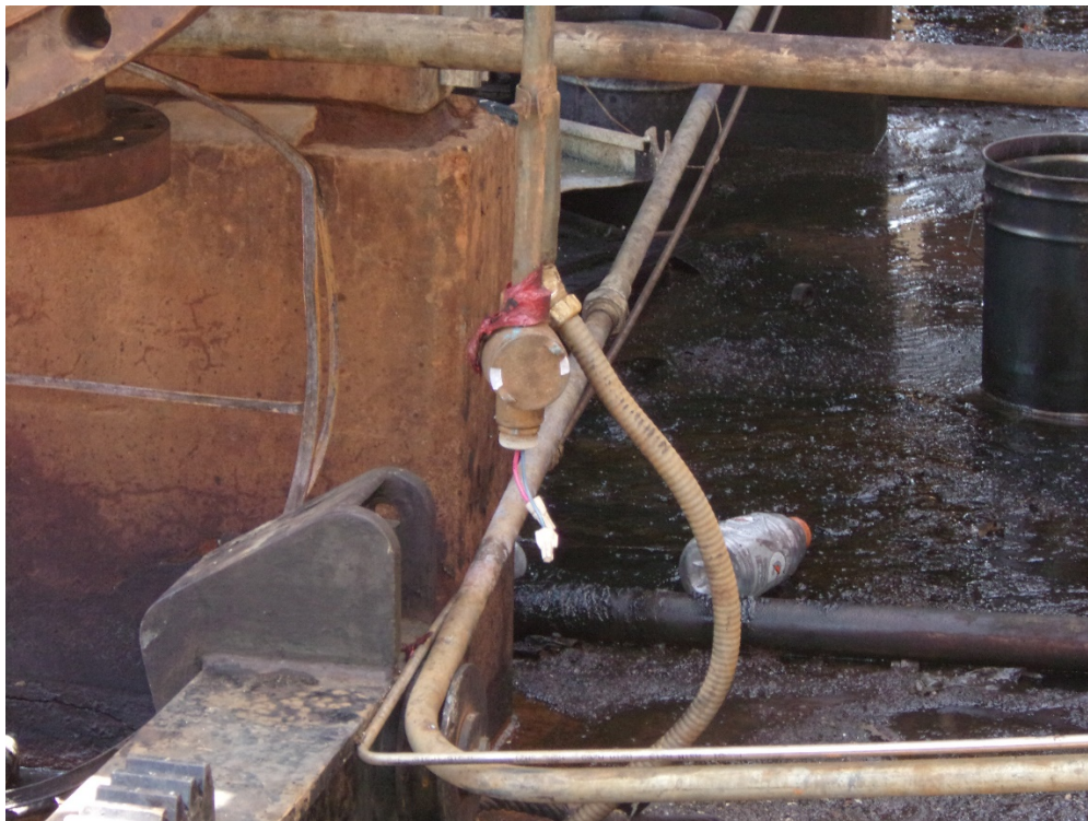
Figure 4. Broken Conduit with Wiring Protected after Fire
