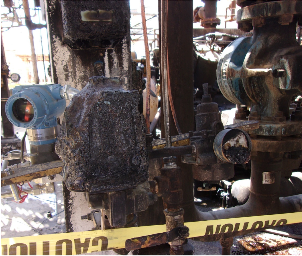
Figure 1. Damage to Instrumentation
