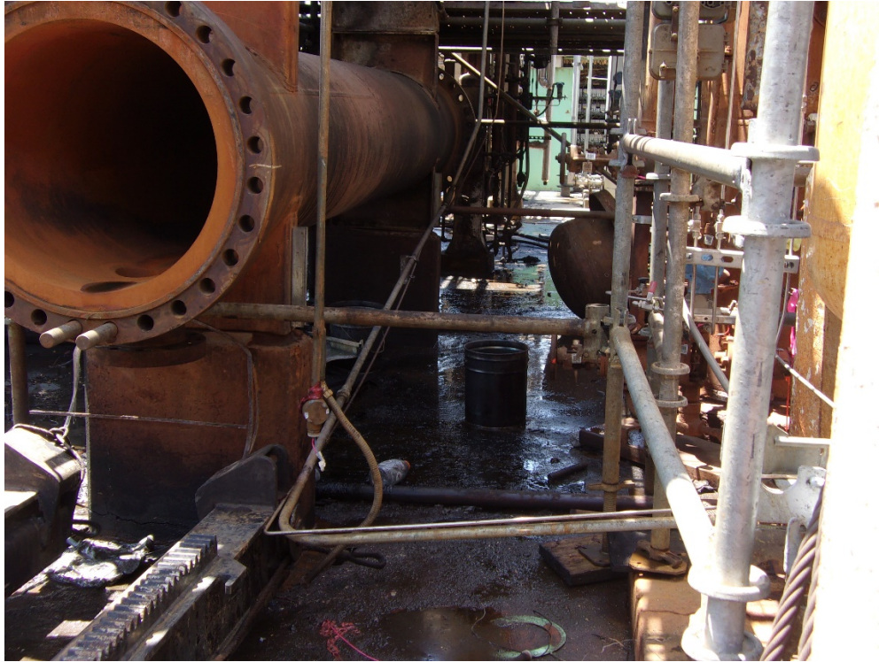
Figure 3. Heat Exchanger Tube Bundle Puller beside Broken Conduit
