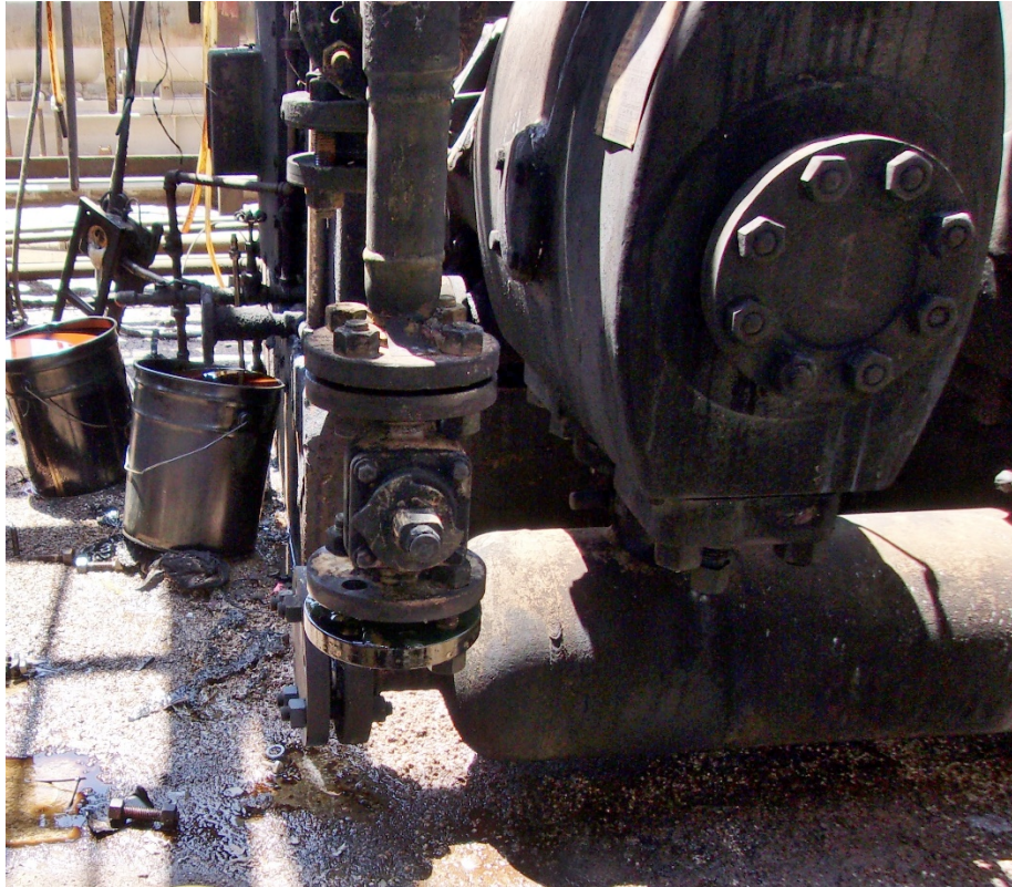
Figure 5. Flare Header Drain Valve by Compressor 3528.07
